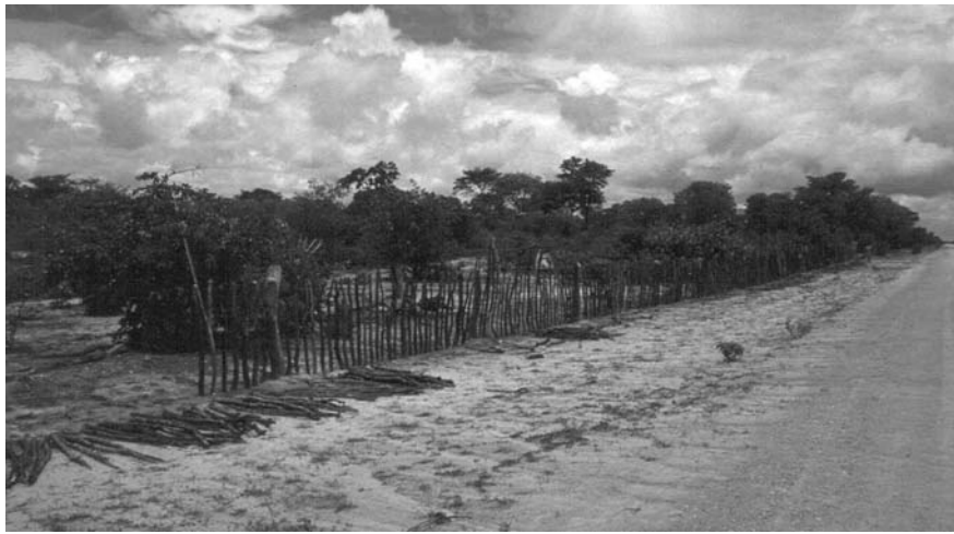
Photo 8: A "modern" 4-strand wire fence in construction. The average dropper spacing is 20 cm!
