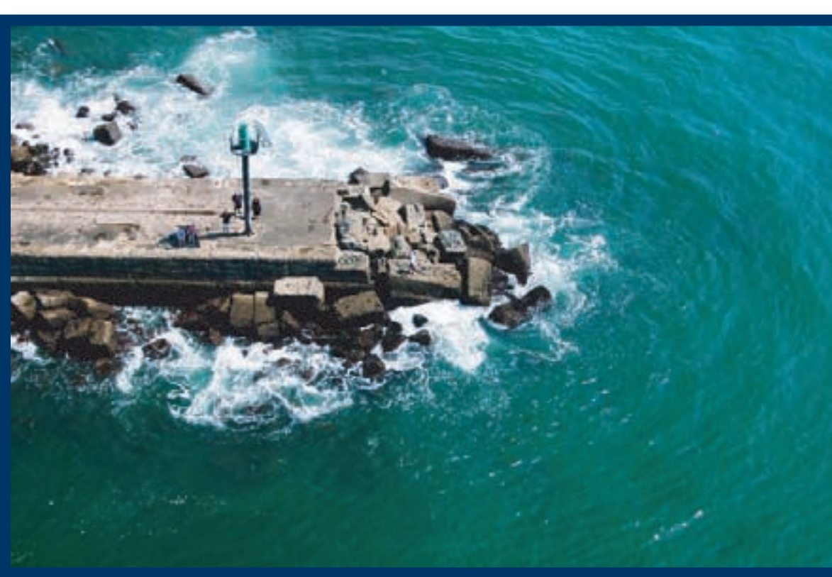
Figure 2: Present SA example of breakwater maintenance required. (Photo: D Phelp)
